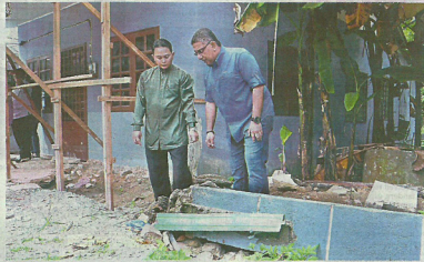
Alaudin (left) showing Hudaib some of the damage done to his house to make way for repair works on a burst pipe in front of his home. Senator Datuk Megat Zulkarnain and Gombak MP, Irwan Dainik.
